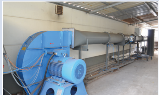
Test station at JASTA-ARMATUREN
